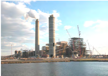
Cross Generating Station – South Carolina Public Service Authority (Santee Cooper) - 600 MW coal-fired units at the South Carolina site
